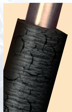
Cracked & Brittled Normal Tube
